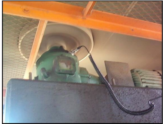
Figure 1: Heat Exchanger Fan analyzed
